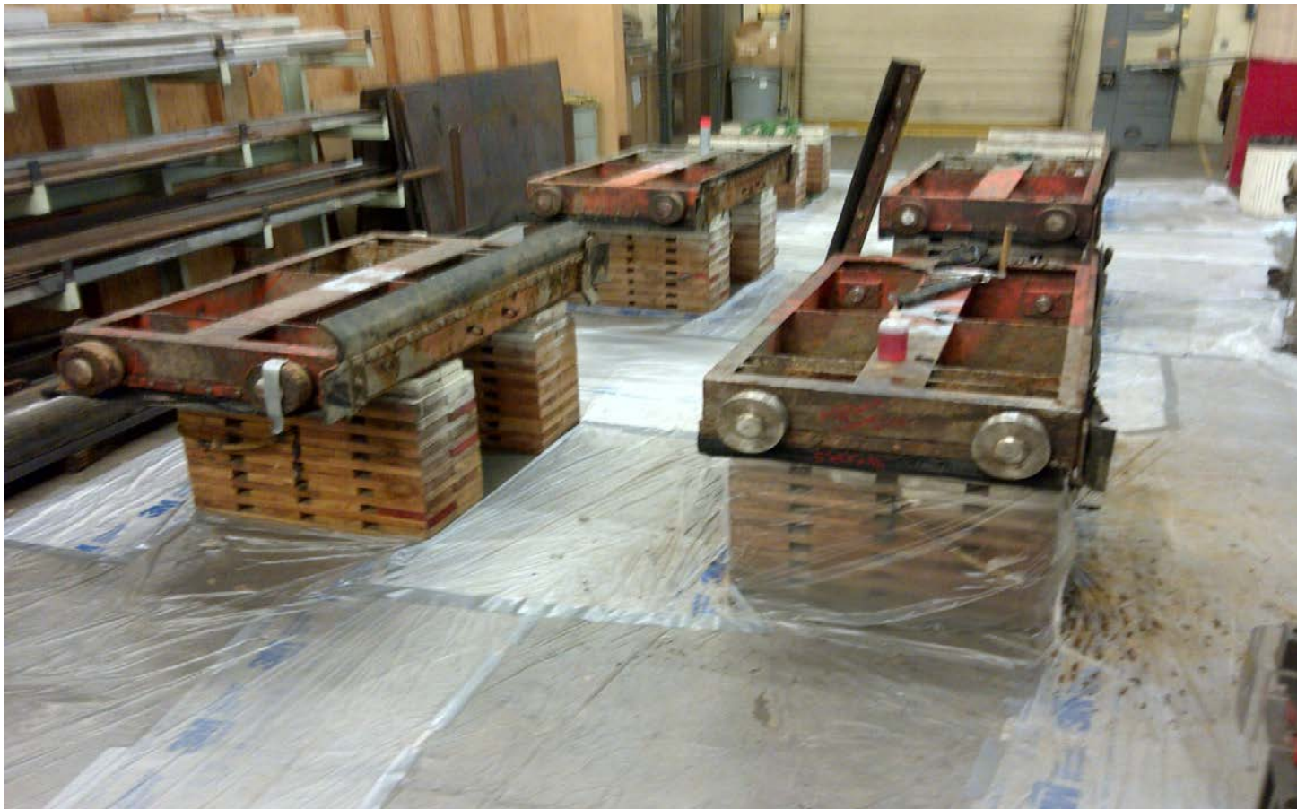
Rehab work on east exit 159 weirs. Upon removal, found in worse condition than expected. Wheels and seals to be replaced. Also wear guide wear to be repaired.
